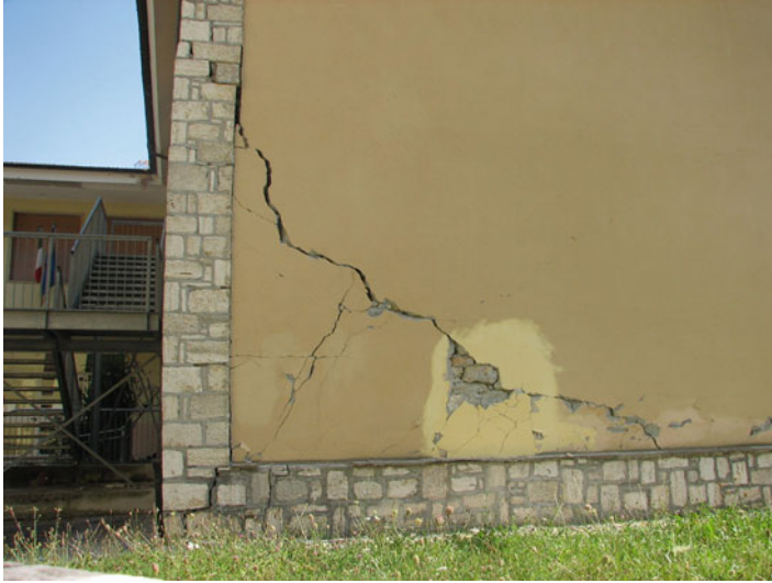
Fig. 20.24 Settlement of the foundations, Arquata 2016
