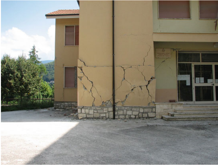
Fig. 20.22 Diagonal cracks due to shear strain, Arquata 2016
