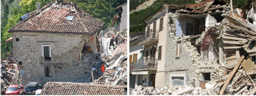
Fig. 20.38 Combined overturning of a multi story wall, Pescara del Tronto 2016
