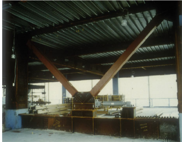
Fig. 17.19 Sumimoto friction dampers installation at Asahi building in Tokyo, Japan
