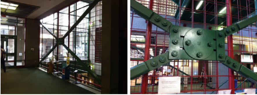
Fig. 17.17 Pall friction dampers installation at the Concordia University library building, Montreal
