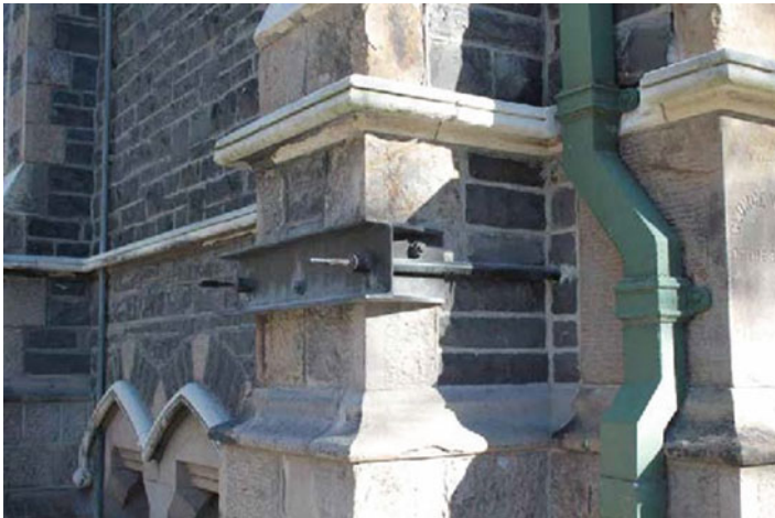
Fig. 20.54 Horizontal post tensioned ties in a masonry building in Christchurch that withstood the 2011 earthquake
